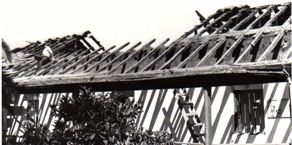
Figure 15. The San Francisco Church after the fire (1983).
