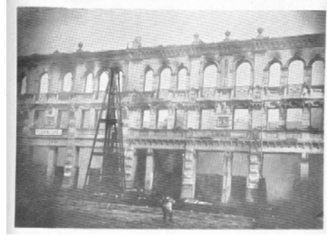
Figure 13. Fire damage of a good construction 3-storey building at a fill soil zone, showing no cracks by the 1906 earthquake. Blanco Street. (Hardy, 1906).
