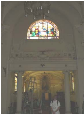
View of the West apse: some diagonal shear cracks are present, starting from the openings area
