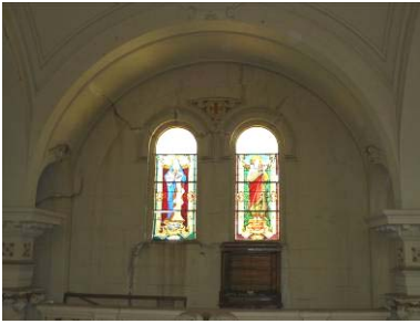
View of the lateral walls of the main nave: some diagonal cracks are present, starting from the openings
