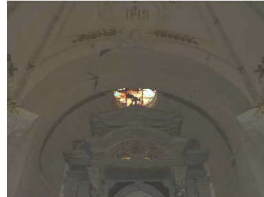
View of the triumphal arch between the presbytery and the South apse: some longitudinal and radial cracks, related to an in-plane seismic action, are present
