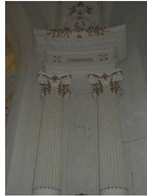
View of the presbytery's columns that support the main dome: no particular cracks are visible on these structural elements
