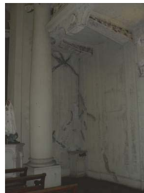
View of the wall that separates the main nave and the presbytery: some diagonal cracks are present in this corner
