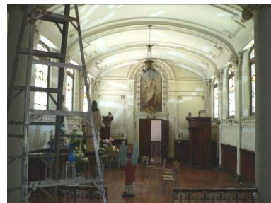
Internal view of the West apse: some cracks are present even in the covering vault
