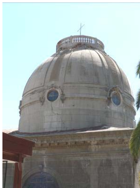
View of the main dome of the church: some diagonal cracks are visible near the round openings, probably due to torsional effects
