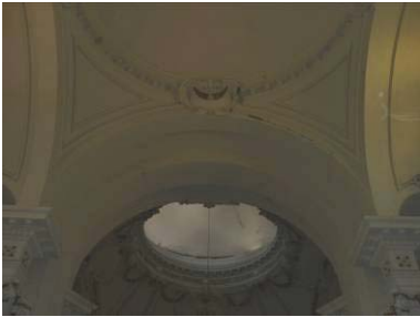
View of the triumphal arch between the main nave and the presbytery: some longitudinal and radial cracks, related to an in-plane seismic action, are present
