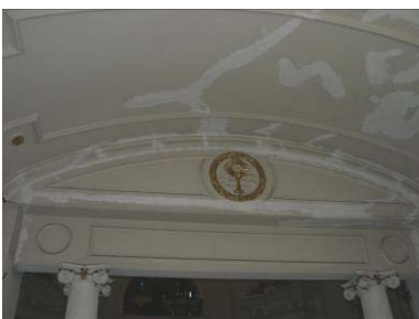
Internal view of the West apse: some cracks are present even in the covering vault
