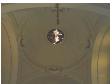
View of one of the two domes of the main nave: no particular cracks are visible on these structural elements
