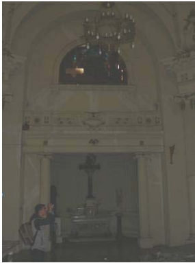
View of the East apse: some diagonal shear cracks are present, starting from the openings area
