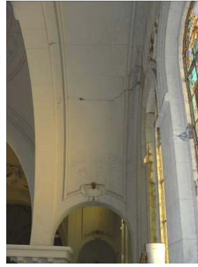
View of one of the lateral arches of the main nave: some radial cracks are present
